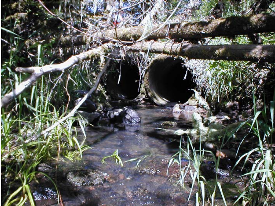
Photo 10. Culvert 12, located on a tributary to Johnson Creek. This is an example of crossing with multiple culverts that both meet ODFW criteria with a culvert gradient of less than 0.5% and a jump height into the culvert of less than 6 inches.
