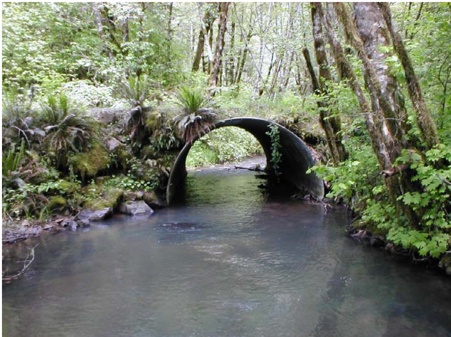
Photo 11. Culvert 323, located on the west fork of Brush Creek. This embedded culvert is an excellent example of a culvert designed to pass juvenile and adult fish. There is no outlet drop and the culvert gradient is the same as the stream channel gradient.
