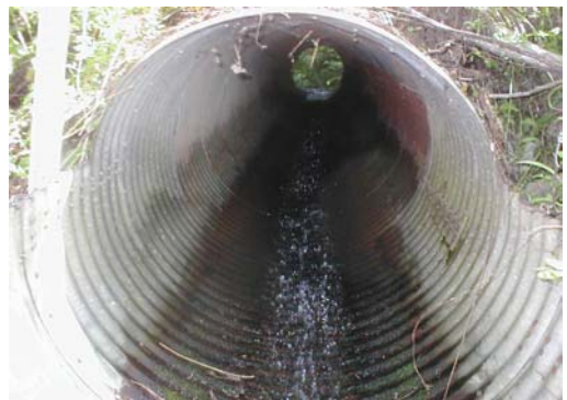
Photo 2. The inlet to a culvert located in the headwaters of Courtney Creek. This culvert has a steep gradient (12%) and shallow water that prevent fish passage.
