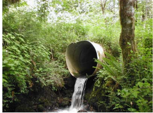
Photo 1. Outlet drop from a culvert located in the headwaters of Brush Creek. This outlet drop is greater than the jumping ability of fish.
